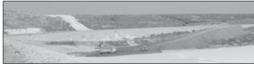
Trucks use new dirt road to carry trash down to bottom of new Cell F.
