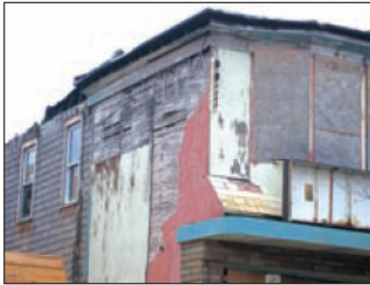
Fire exposed building's ancient lathing.
